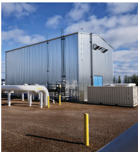
Example of a compressor station
