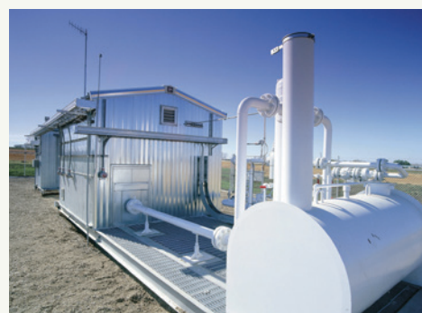
Example of a meter station
