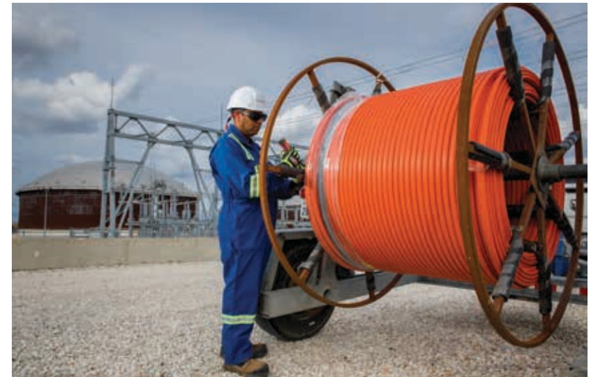
As part of our commitment to innovation, we partnered with HiFi Engineering, Enbridge and the Government of Alberta to pilot new technology that uses fiber optic cable installed along oil pipelines as a highly sensitive vibration sensor, adding another layer to our comprehensive monitoring and leak detection program. Learn more on our website . Keystone Pipeline Terminal, Houston, Texas.
