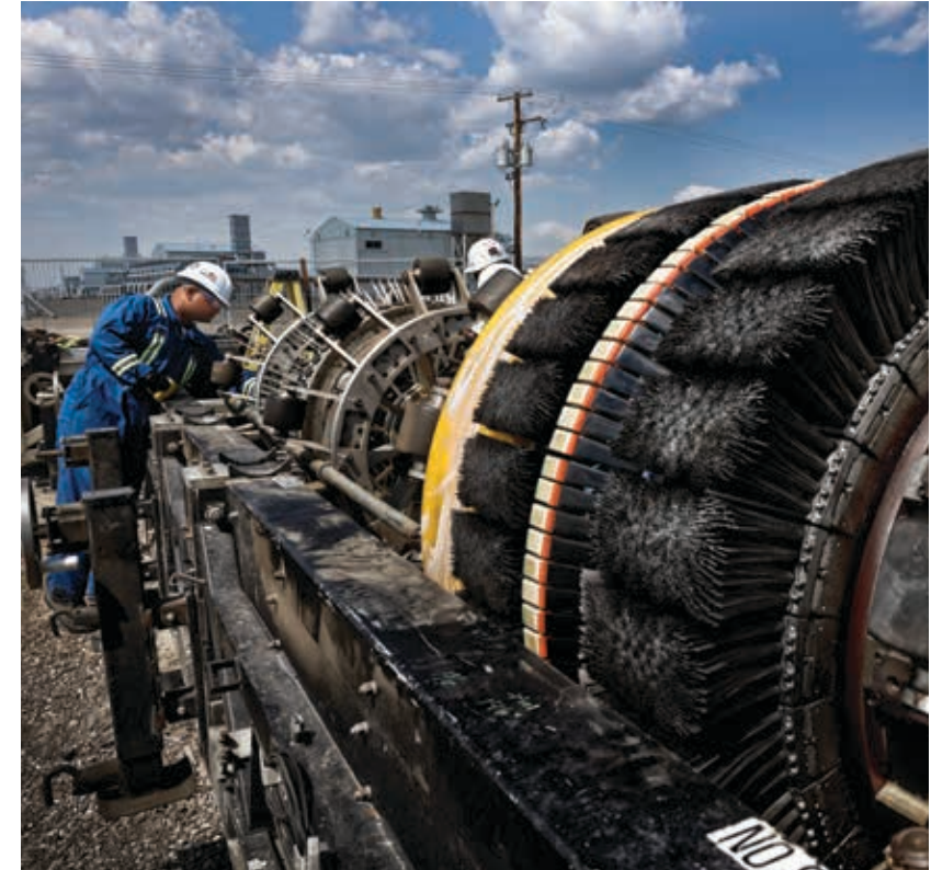
After years of detailed planning and collaboration by a number of groups within TransCanada, our Canadian natural gas pipelines operations team set a new record for completing a, 941-kilometre in-line inspection run on the Canadian Mainline in the summer of 2017. Learn more on our website .
